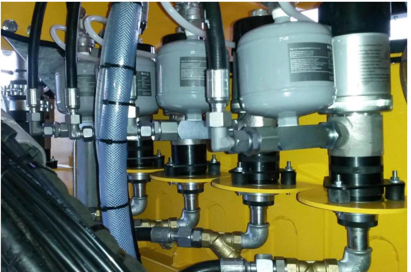
4 units pneumatic operated oil-pumps, approx. 20-30 ltr/min flow-rate
