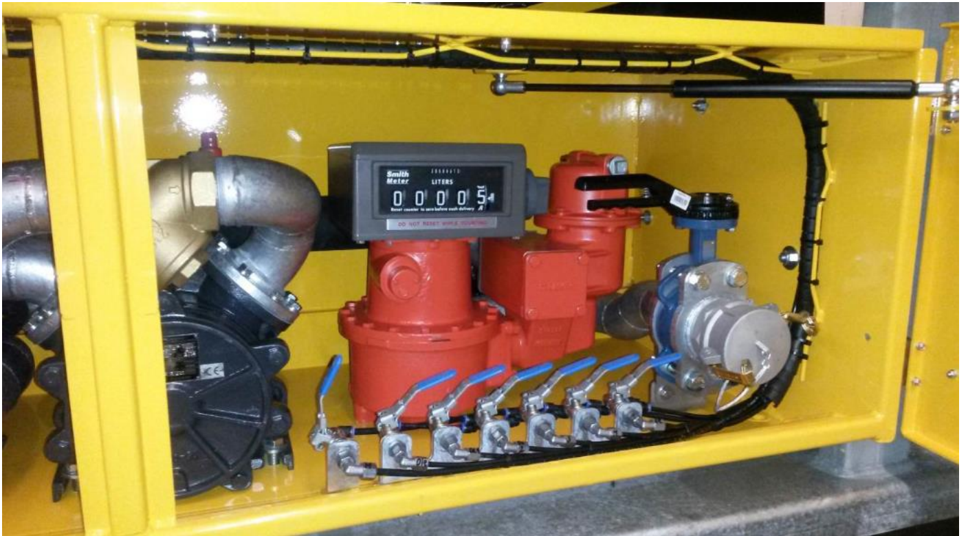
Detail: Right side of the cabinet with pump and metering system
